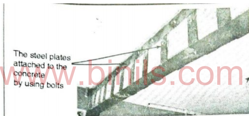
Fig. 6.1.3(a) : The steel plates are attached to the concrete by using bolts
