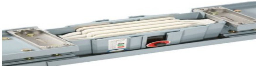
Fig5 cable tray Earthing
