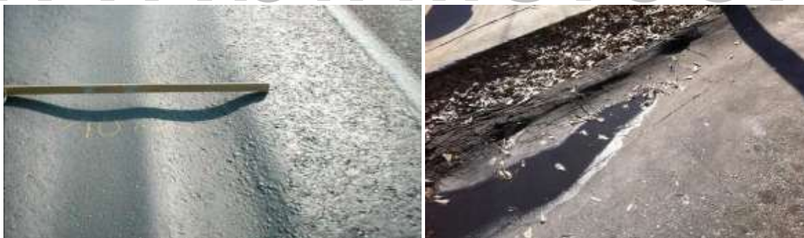
Rutting on Road Surface
