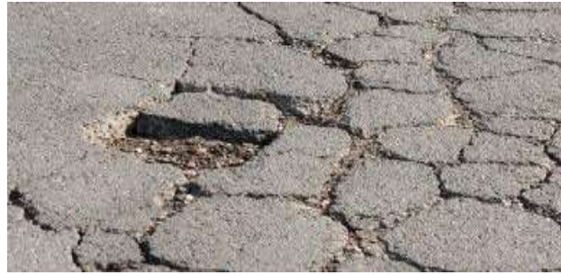
Frost Crack on Road Surface
