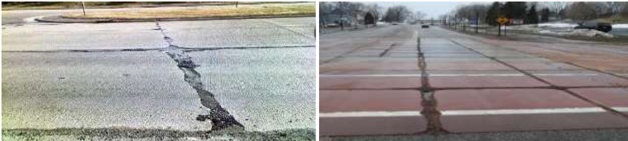
Joint Spalling Crack on Road Surface
