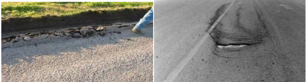
Shear Fail on Road Surface
