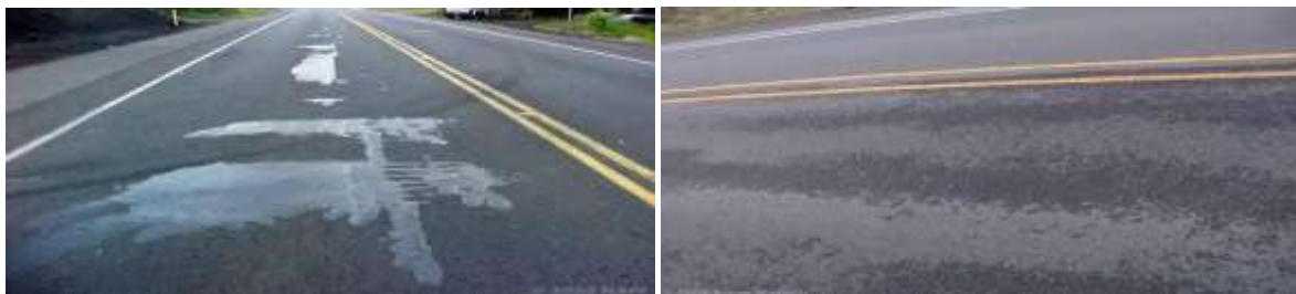
Bleeding Failure on Road Surface
