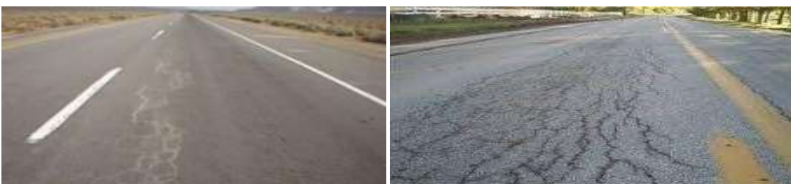
Alligators on Road surface
