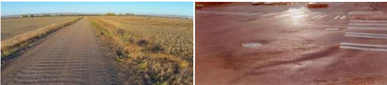
Wave Failure on Road Surface
