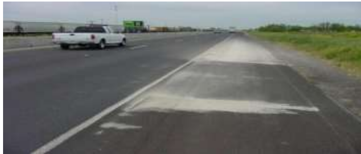
Mud Pumping on Road Surface
