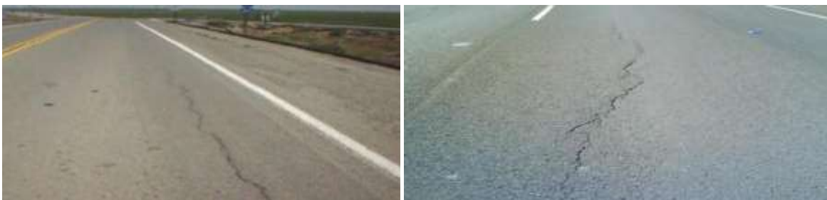
Longitudinal Crack on Road Surface
