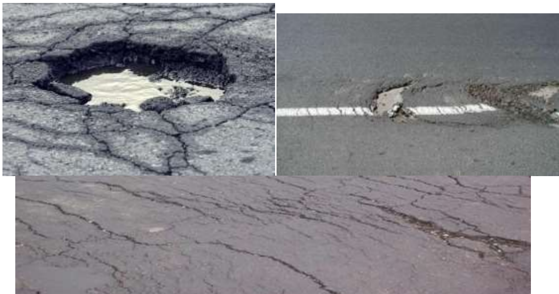
Road Failure due to Lack of Binding
