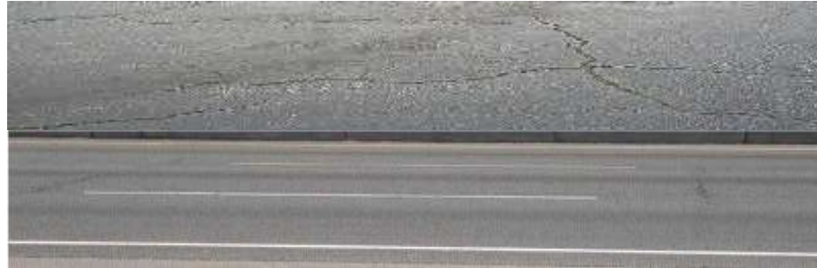
Reflection Crack on Road Surface
